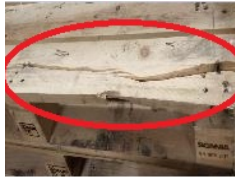
6. Repair, cracked plank
