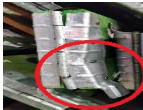
7. Repair, bent corner
