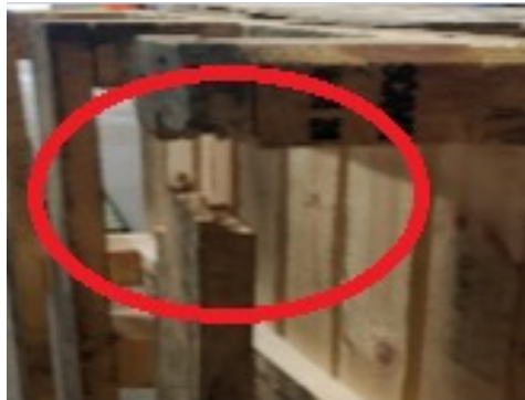
5. Repair, broken runner
