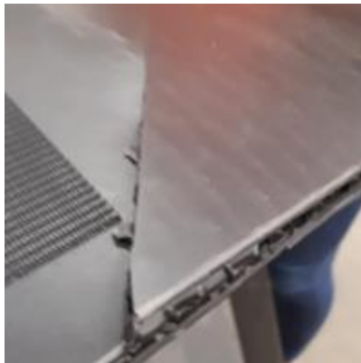
Damage through sleeve
