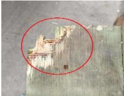
Cracks and damages that might allow water to get inside
