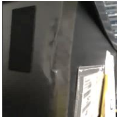
Damage has bended sleeve corner
