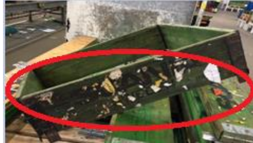
Instable and very rusty
