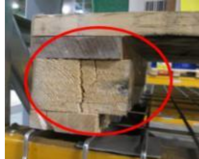
Broken, loose and/or missing Blocks
