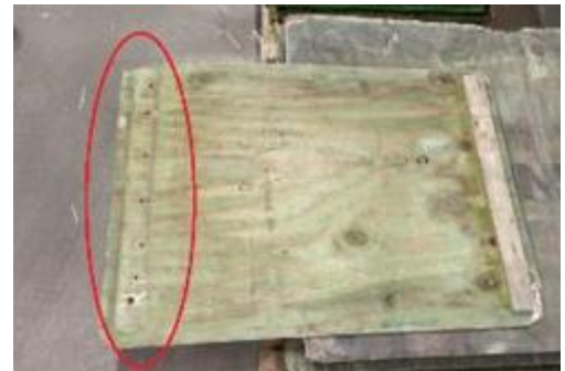
Missing plank, should be repaired.
