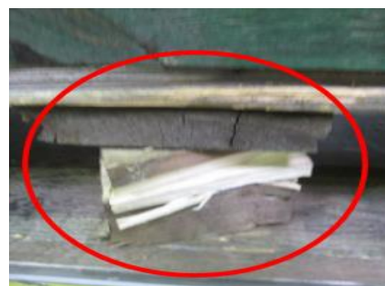
Broken, loose and/or missing Blocks
