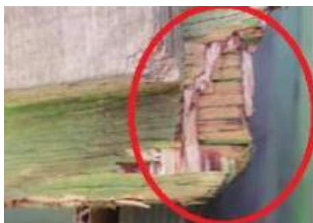
Cracked at the corner
